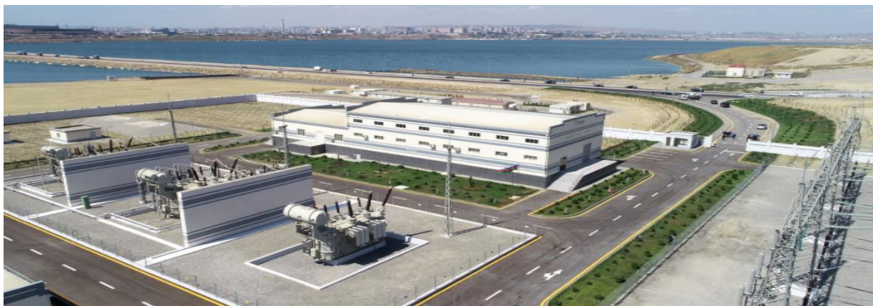
Figure 3.2. The view of Boyukshor substation and Boyukshor Lake [20]
