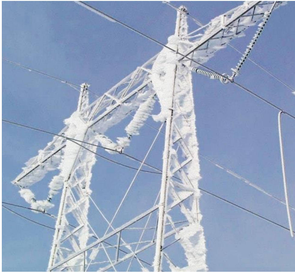
Figure 2.5 Frozen high-voltage transmission tower
