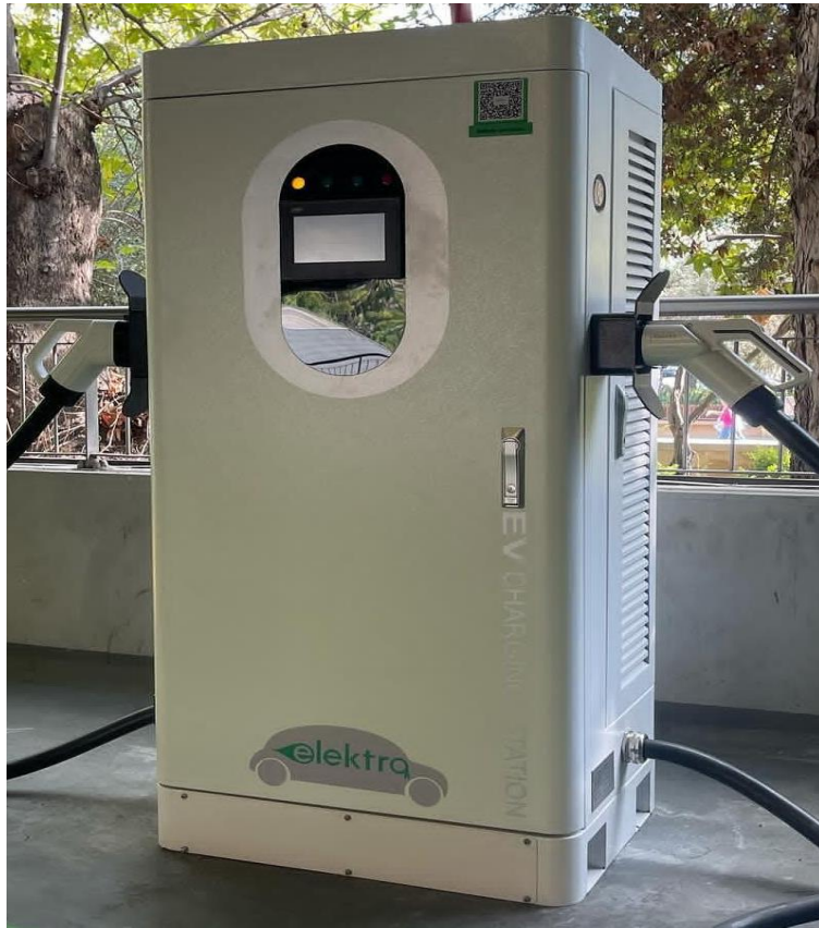
Fig 3.2 120 kW Elektra.az charger
